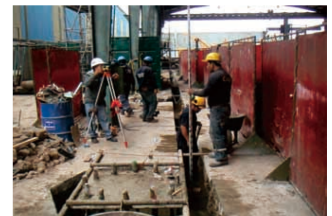
Eight sets jib crane been installed in peru
