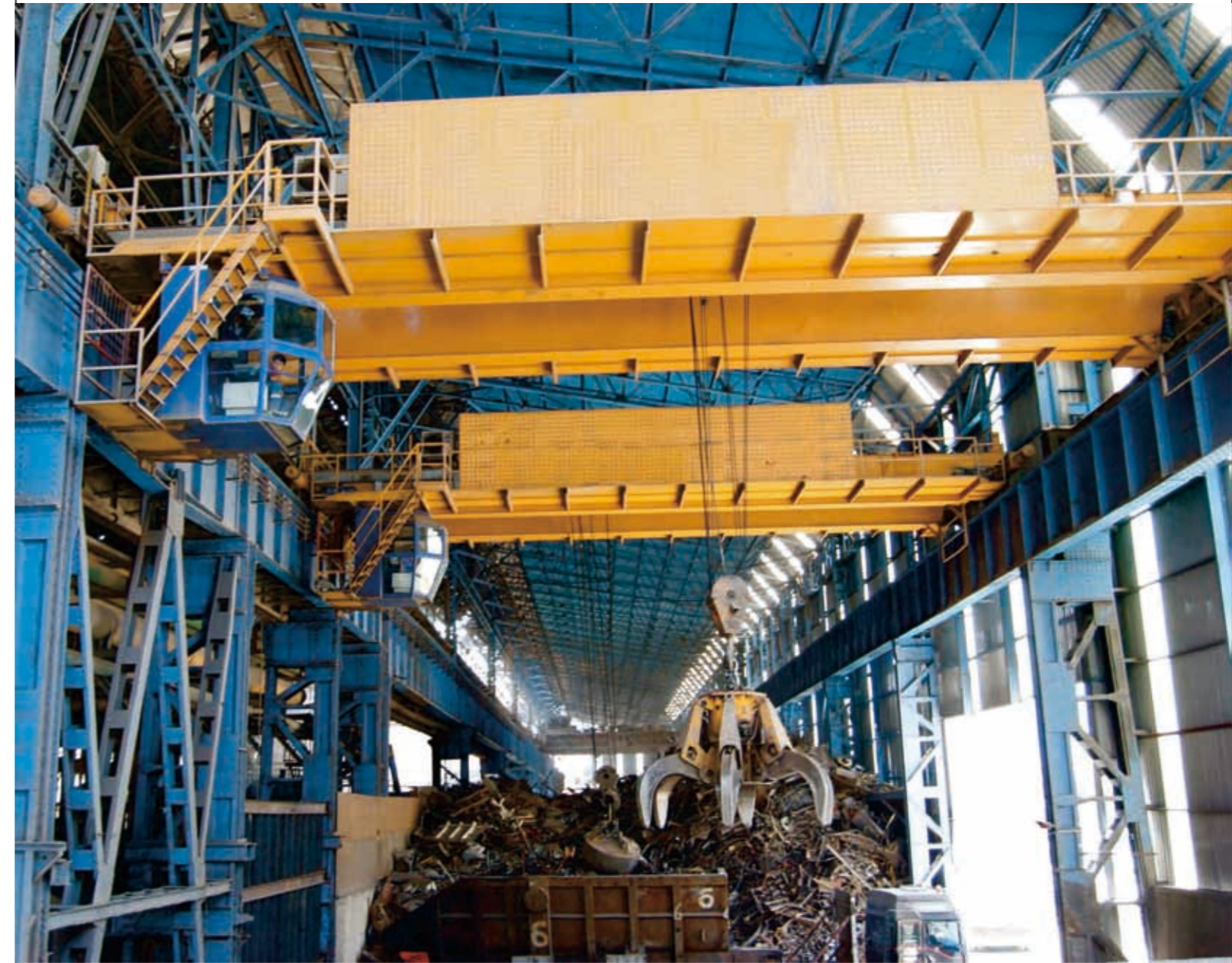
This grab overhead crane installed in our Turkey Customer Factory. ( 20t overhead crane)
